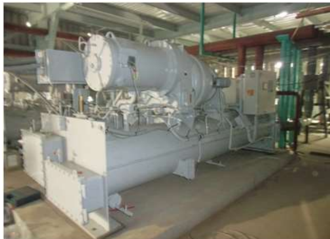
Installed Centrifugal Chiller
