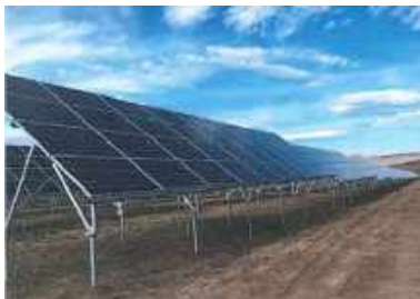
Solar power ,Farmdo Co., Ltd.,Mongolia
