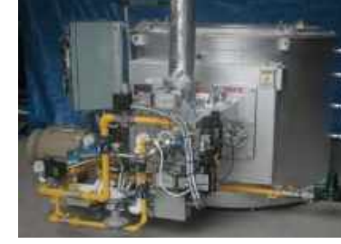
Regenerative Burners in industries, Toyotsu Machinery, Indonesia
