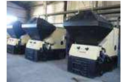
High-efficiency Heat only Boilers, Suuri-Keikaku, Mongolia
