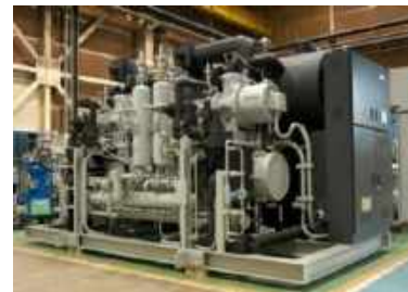
High efficient refrigerator, Mayekawa MFG, Indonesia
