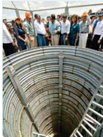
Drainage well for landslides (Honduras)
