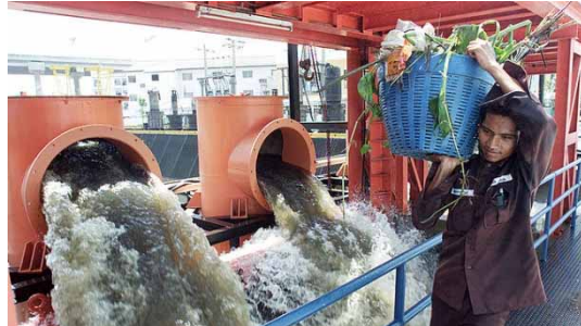
Recovery from wastewater
