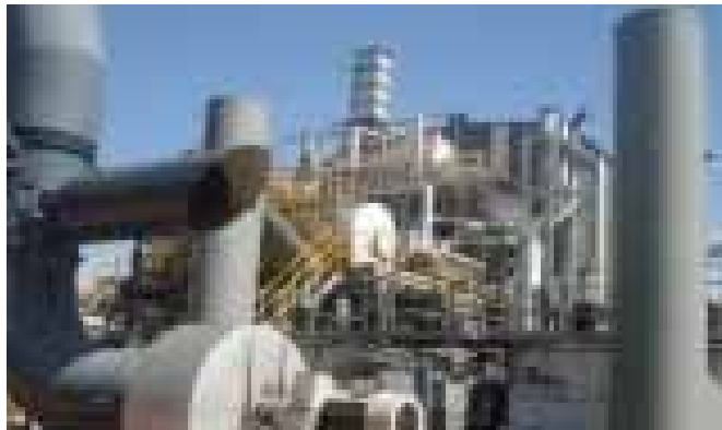
Coal mine methane capture
