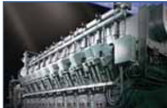
Cogeneration system (Indonesia)
